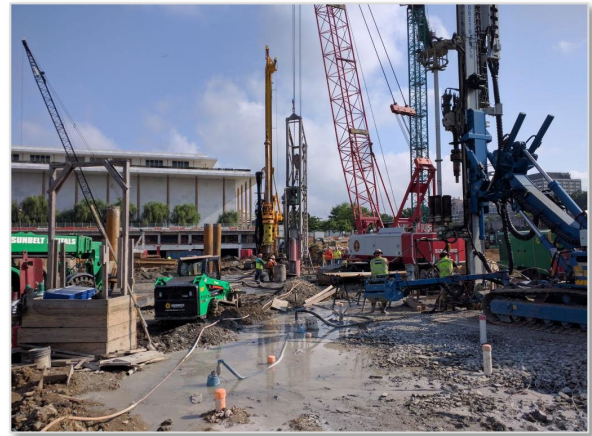
Photo A.16: CSO 021 Diversion Facilities (DC Water photo)
