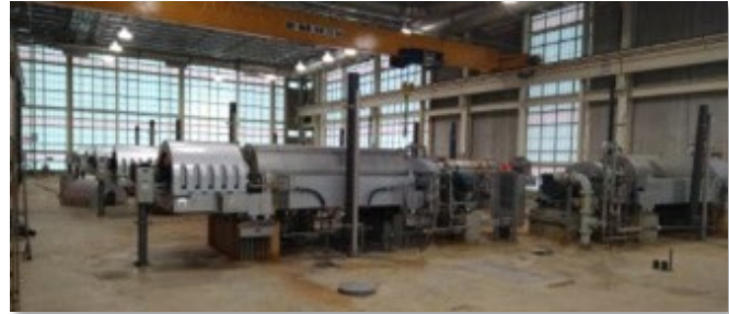
Photo 5-4: Blue Plains AWT Pre-Dewatering Centrifuges (PEER photo)
