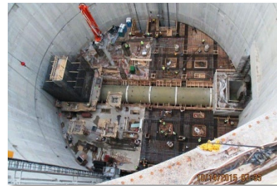
Photo 5-7: Tunnel Dewatering Pump Station (DC Water photo)
