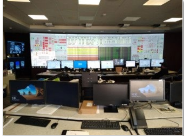
Photo A.5: Blue Plains AWWTP Central – control room (PEER photo)
