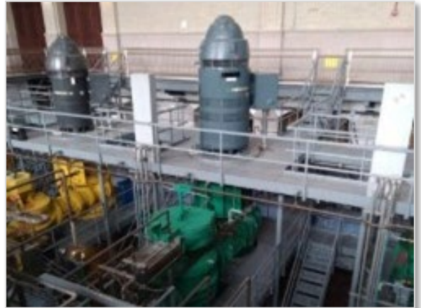
Photo A.2: Bryant Street Water Pumping Station – pump motor assembly (PEER photo)
