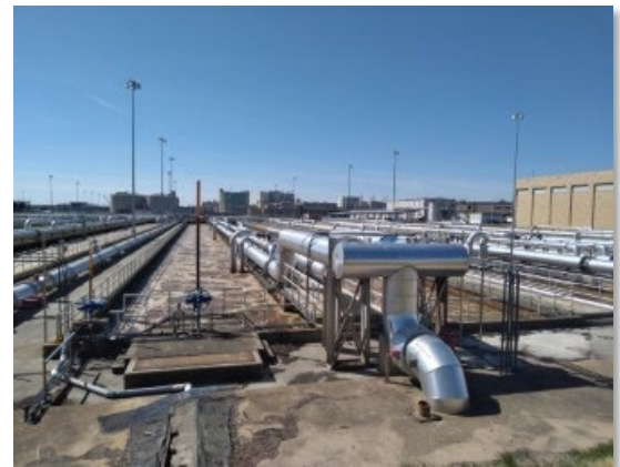
Photo 5-2: Blue Plains AWWTP Secondary Aeration Basin (PEER photo)
