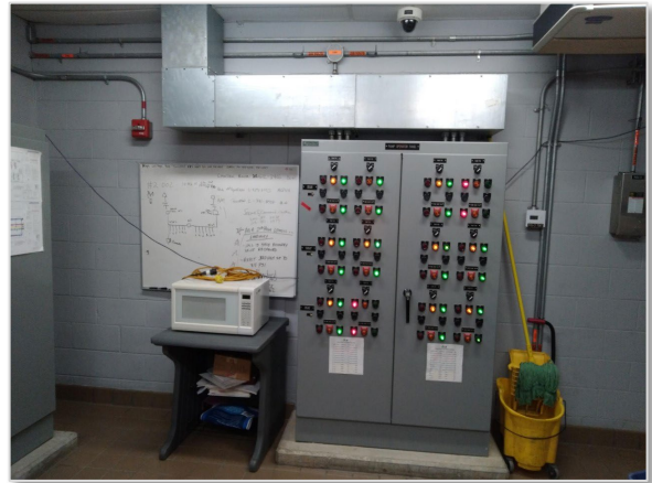
Photo A.3: Anacostia Water Pumping Station – control room (PEER photo)
