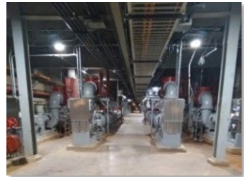
Photo 5-3: Blue Plains AWWTP Nitrification Return Sludge Gallery (PEER photo)
