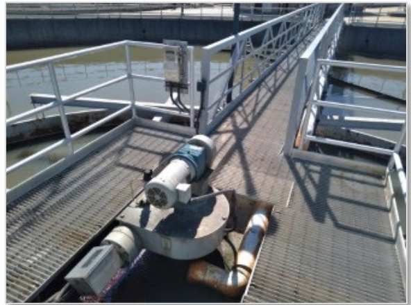
Photo A.7: Blue Plains AWWTP Primary Clarifier – drive unit (PEER photo)
