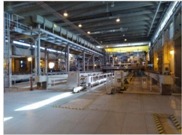
Photo A.6: Blue Plains AWWTP Raw Wastewater Pumping Station-1 – screening room area (PEER photo)
