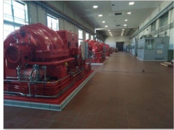
Photo A.8: Blue Plains AWWTP Secondary Blower Building – blower room (PEER photo)
