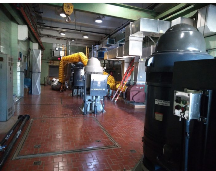
Photo 5-9: O Street Pumping Station Pump Room (PEER photo)
