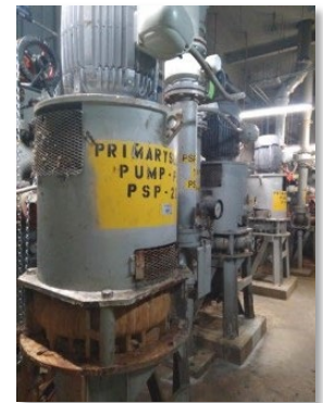
Photo 5-1: Blue Plains AWWTP Primary Sludge Pump (PEER photo)
