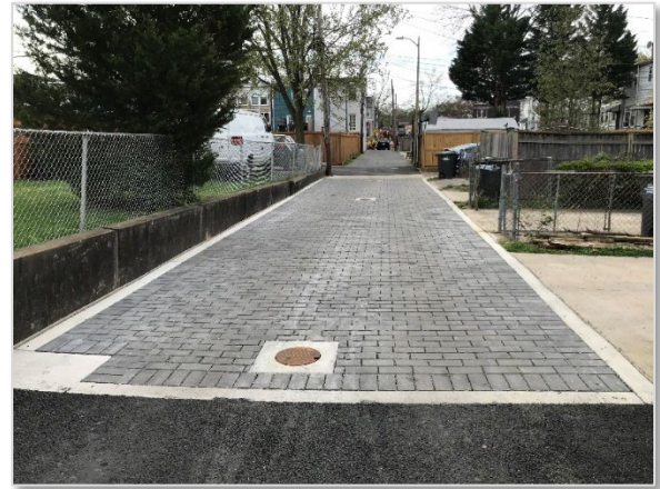
Photo A.15: Rock Creek Project B – permeable pavement installed in an alley (PEER photo)
