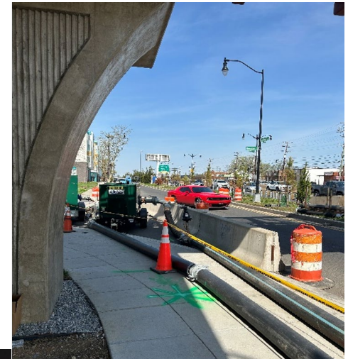
Figure 1. Sewer Failure Location (green asterisk) and bypass pumping.
