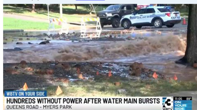
Recent pipe failure in Charlotte
