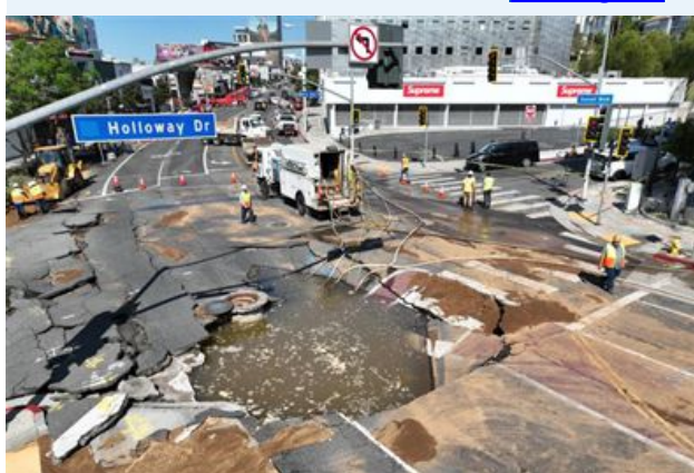
Recent transmission main failure in Los Angeles
