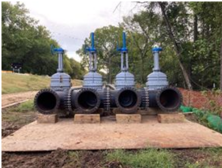
Bypass Pipe Manifold
