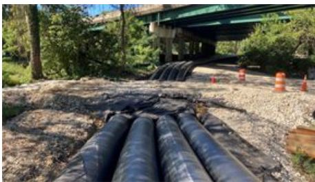
Bypass pipe crossing
