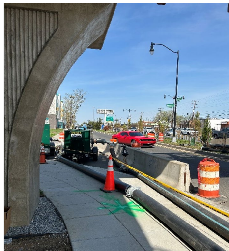
Figure 1. Sewer Failure Location (green asterisk) and bypass pumping.
