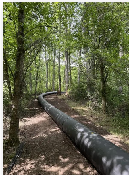
Muddy Branch MH410 to 411
