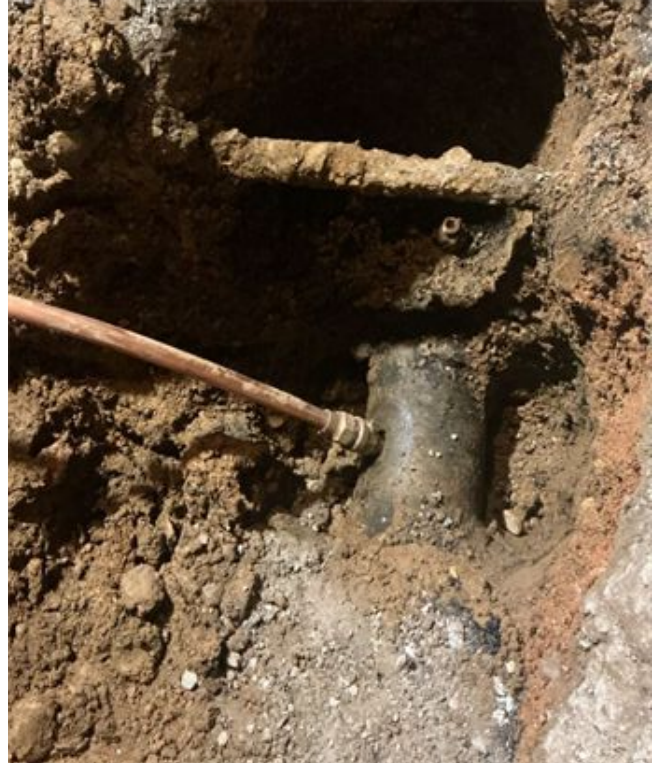
New Copper Service Line Tap
