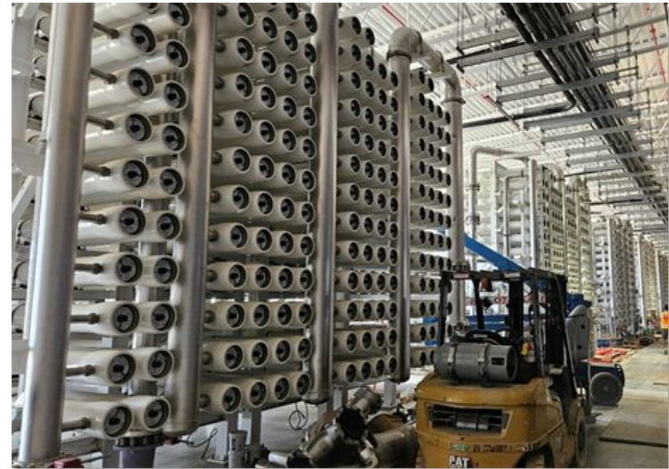
North City Pure Water Facility, San Diego CA
