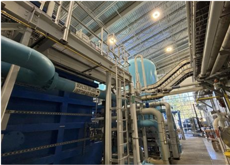
HRSD SWIFT Research Facility, Suffolk, VA
