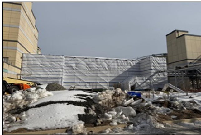
Blue Plains AWTP Cambi system emergency response
