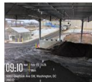
Biosolids Curing Pad in Use
