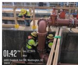
SWPS Piping Discharge Modifications
