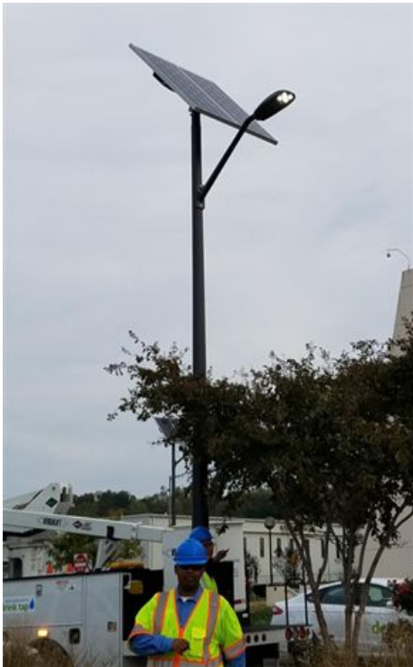
Central Ops Facility Lot Lights 550 kWh/mo originally (24 units) 150 kWh/mo now (6 units)
