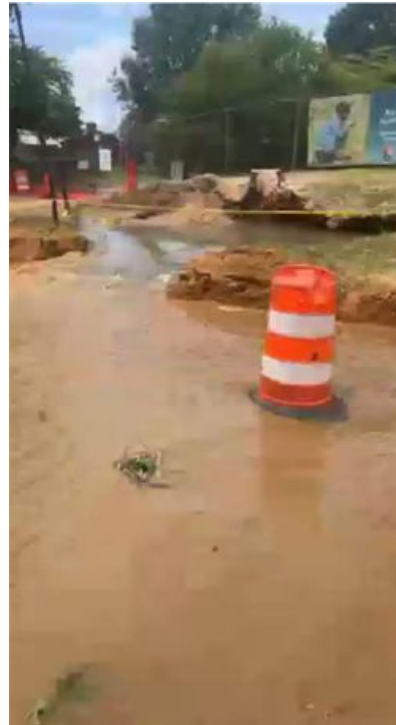
July 21 st - Sanitary Sewer Overflow
