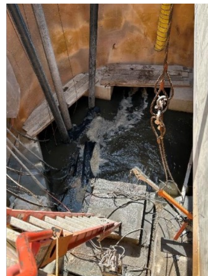
Flow Conversion at MH-31
