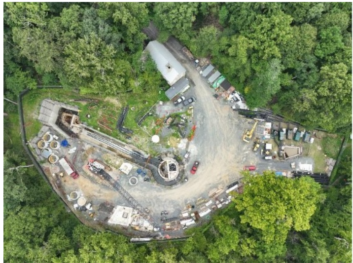
Flow Conversion at MH-31
