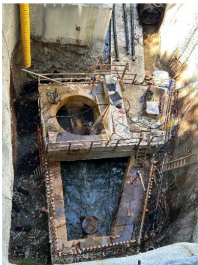
Flow Conversion at MH-30.59
