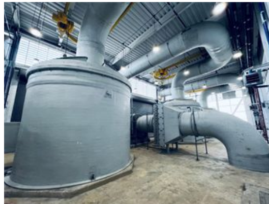
W Street - Ventilation Control Facility
