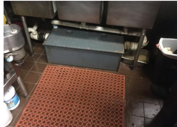
Grease trap under sink
