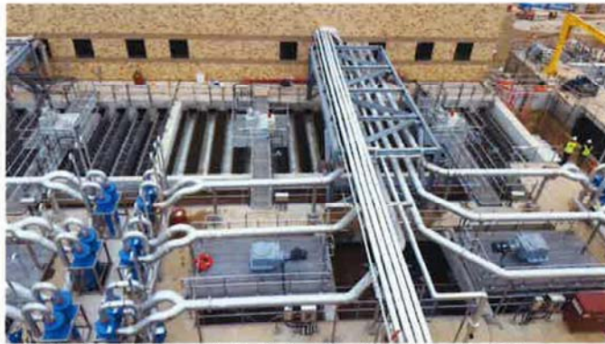
Aerial view of the High Rate Clarification (HRC) process
