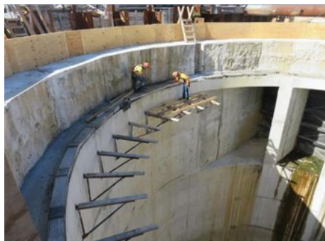
Drop Shaft Internals
