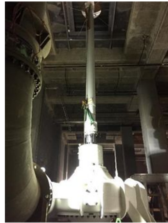
Tunnel Dewatering Pump
