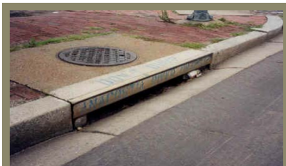
Catch basins can fill with trash.
