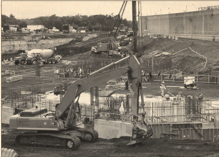
Work on the Enhanced Nutrient Removal Facilities (ENRF) began in 2011 and is due to be completed in 2014. It is just one of three massive construction projects on Blue Plains.
