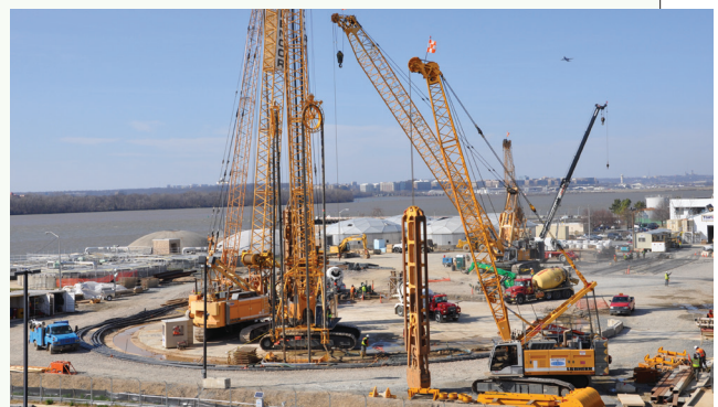
The first portion is called the Blue Plains Tunnel. Here construction begins at Blue Plains to build the shaft nearly 16 stories deep where the tunneling will begin.
