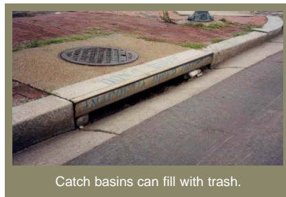
Trash on street washes into catch basin.
