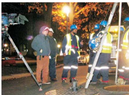
Crews from the History Channel and WASA Sewer Services film underground Tiber Creek sewer.
