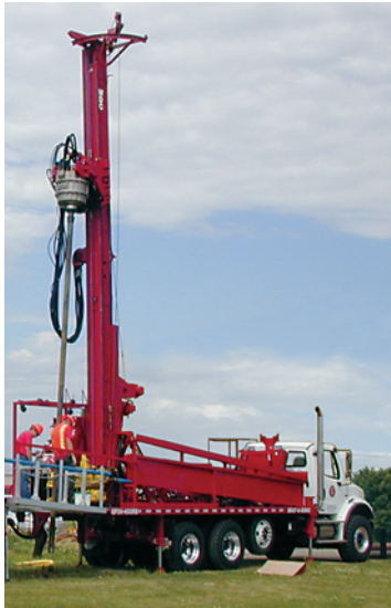
Sonic drilling rigs, like this one, will be in District neighborhoods along prospective tunnel routes to collect soil samples between 150–250 feet deep.
