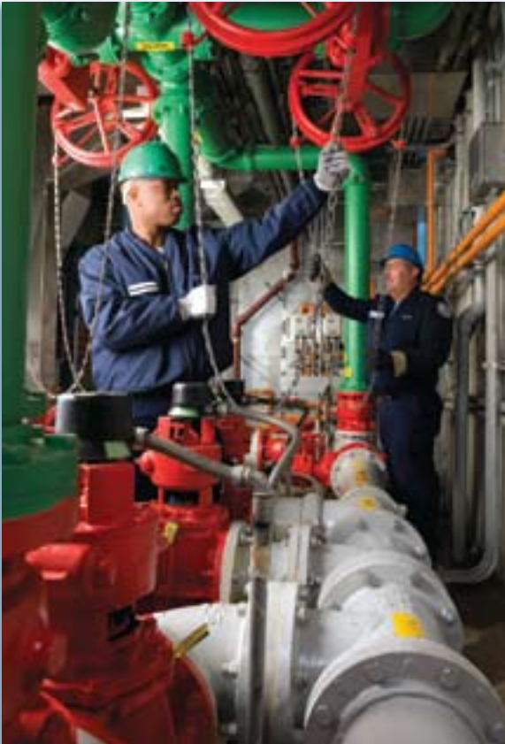
Operators at Blue Plains sludge pumping station are changing the flow direction by turning large overhead valves connected to chains.
