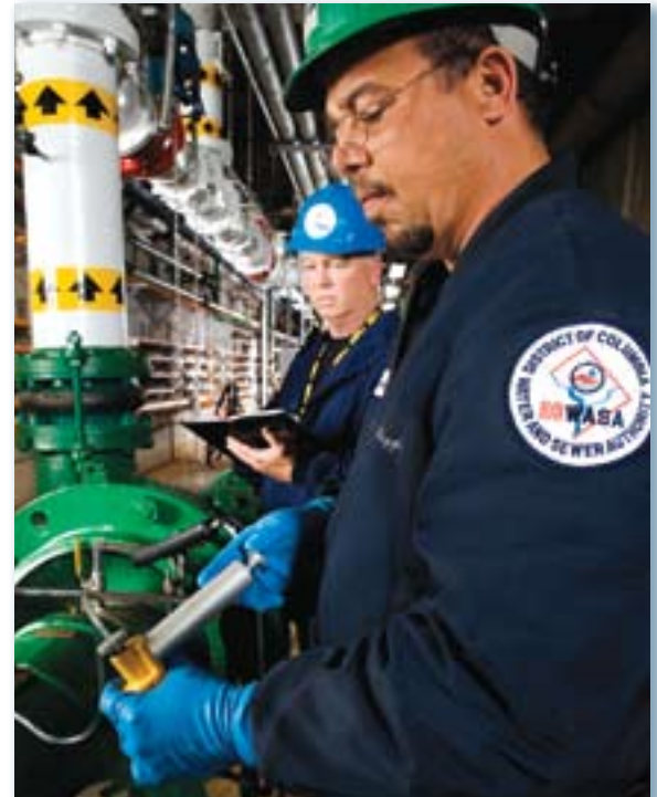
In the plant's dewatering grit chamber, vibration and oil analyses determine the amount of wear on the pumps.
