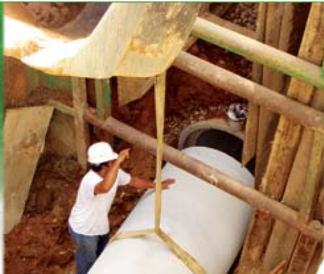
(Left) Stormwater pipe upgrades improve drainage of new development in the District.
