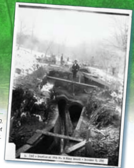
The existing sewer system dates back to 1810. (Right) Building a sewer overflow at 14th Street and Piney Branch, NW, on December 8, 1893.
