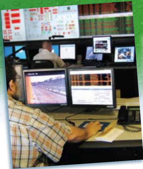
(Left) This Central Control Room at Blue Plains controls and monitors the processes and equipment at the wastewater treatment plant.
