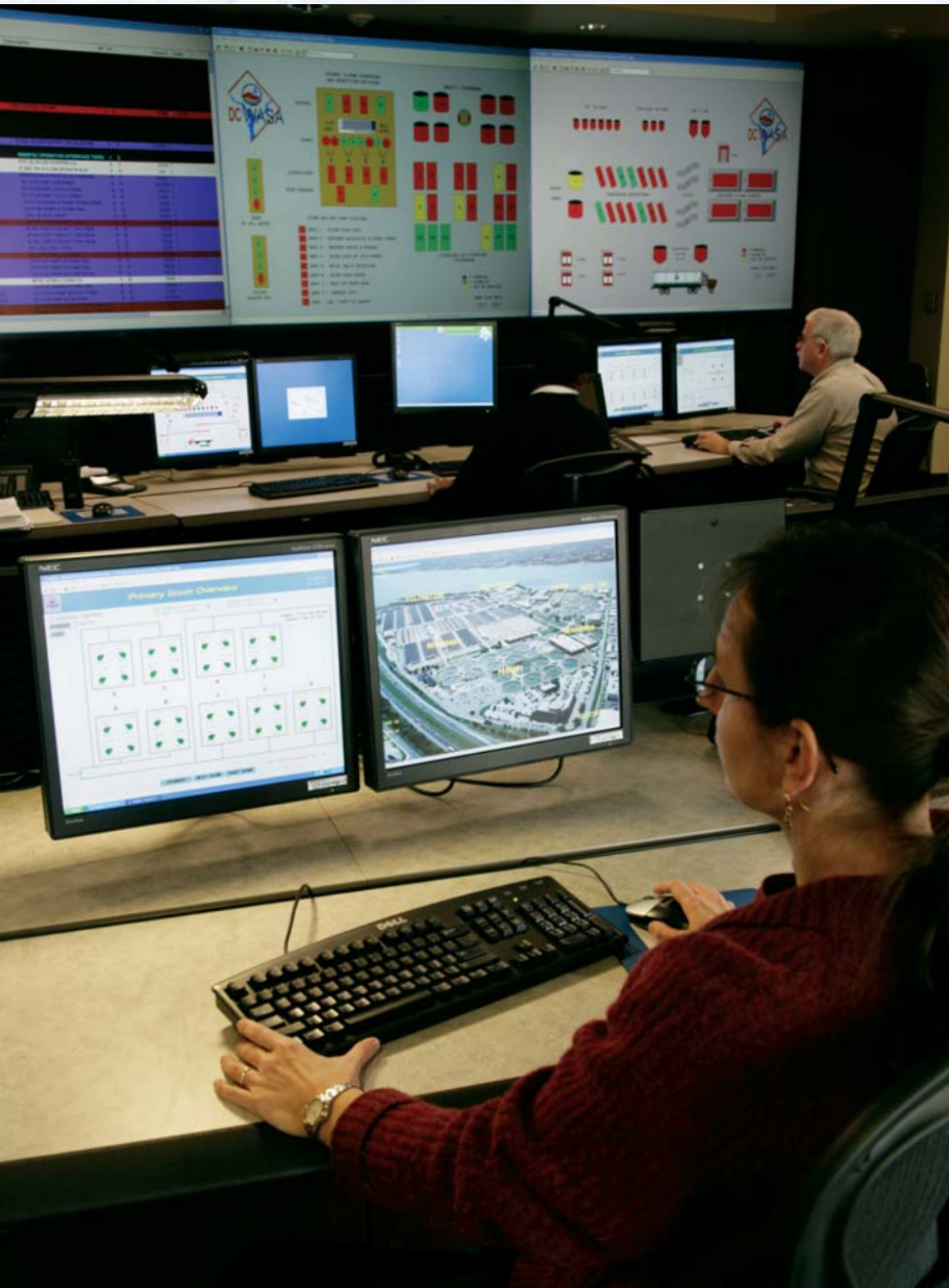
The Central Control Room at Blue Plains is where vital aspects of the treatment process and related equipment are monitored and controlled 24 hours a day.
