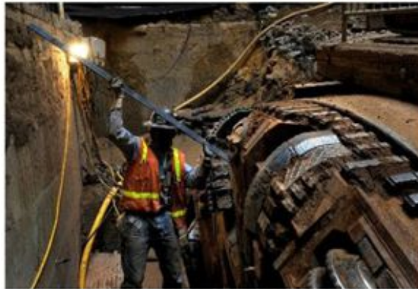
The bits (foreground right) can be seen on the disk cutters on the face of the huge boring machine that is making a tunnel under the Anacostia River. Buck Price hands a rod to a co-worker inside the boring machine. (Michael S. Williamson/The Washington Post)
