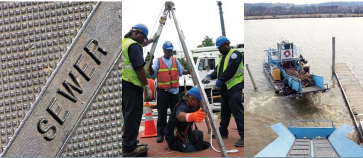
ABOVE: In addition to work on pipelines and pumping stations, sewer services includes the operations of skimmer boats, which remove an average of 400 tons of floating trash and debris annually from the Anacostia and Potomac rivers.
