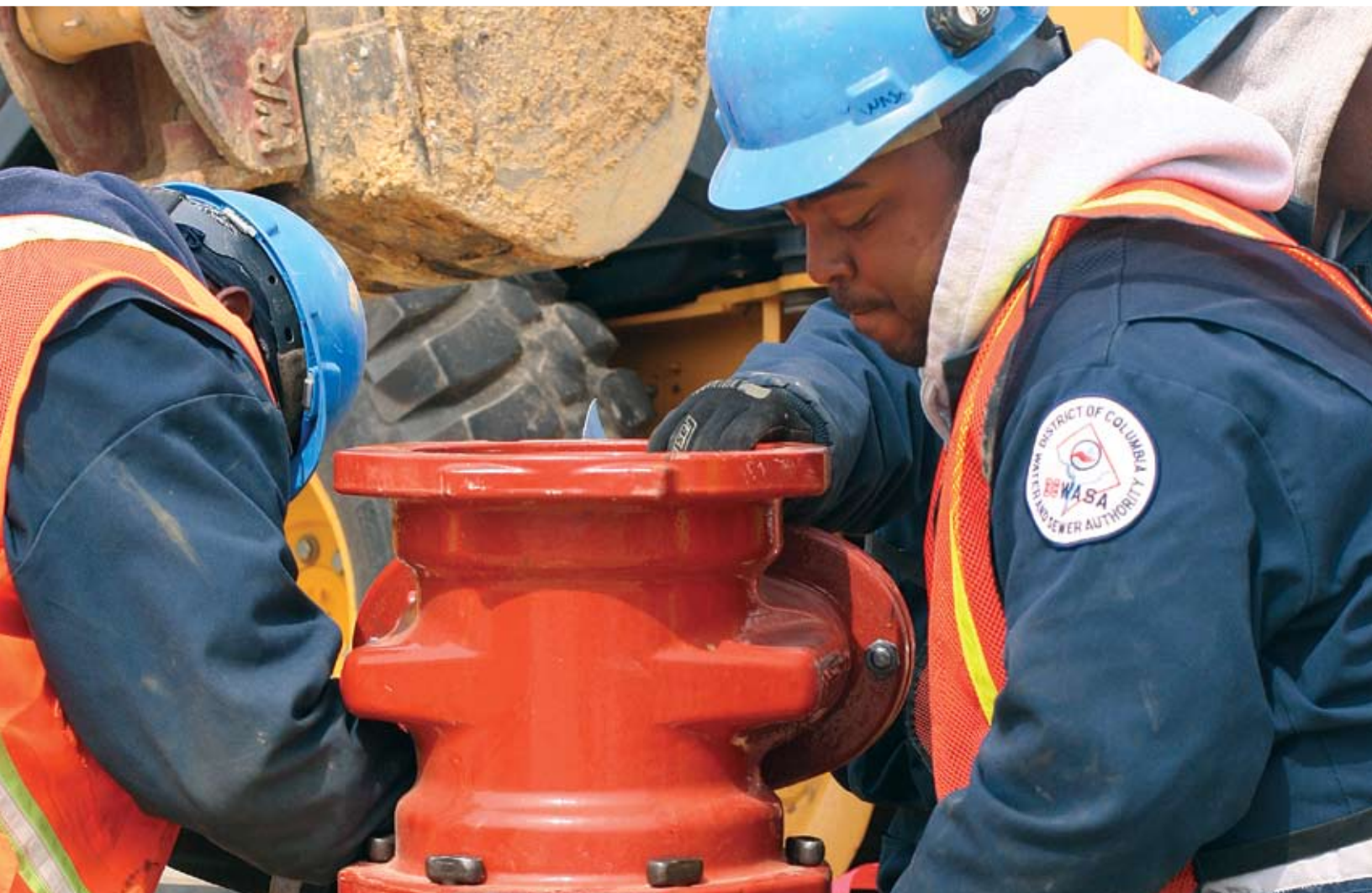
ABOVE: The replacement and rehabilitation of mains and valves is an ongoing program to improve the reliability of the water distribution system.
