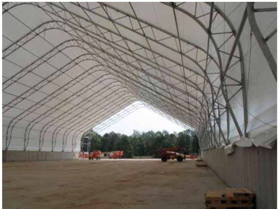
A state-of-the-art indoor storage facility built by Nutri-Blend will allow all trucks to unload inside and will treat all building air through a biofilter for odor control.
