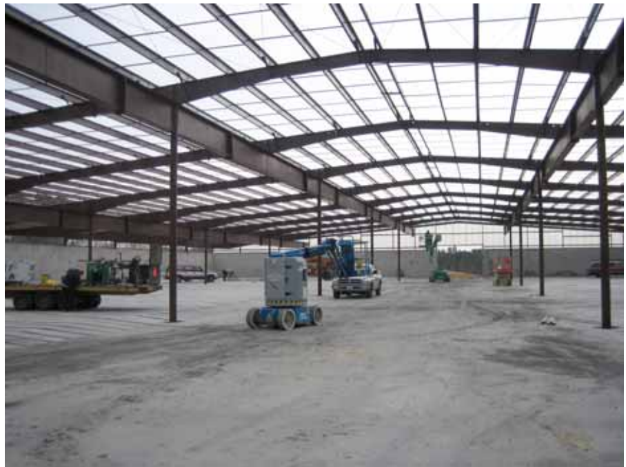
McGill Environmental Systems of NC Inc. began constructing a composting facility in Waverly, VA to provide year-round biosolids and other feedstock processing. The facility is expected to provide another option for DC-WASA residuals processing when it begins taking material in 2008.
