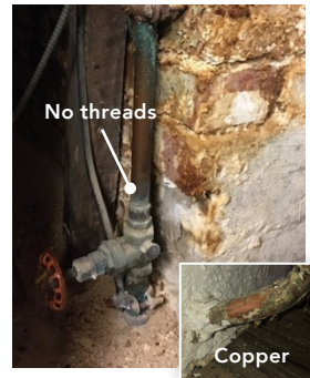
No "threads" on copper pipes. Green color is copper corrosion.
