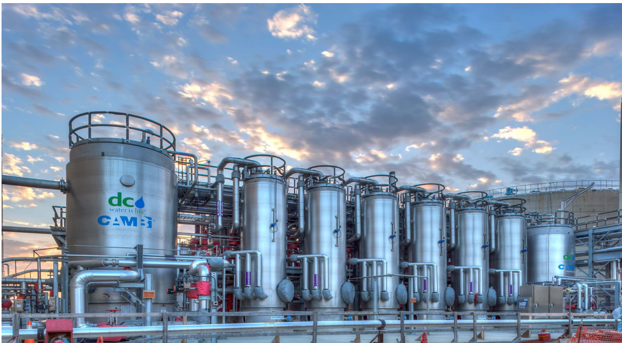
The Cambi Thermal Hydrolysis Process (THP) at the Blue Plains Advanced Wastewater Treatment Plant
