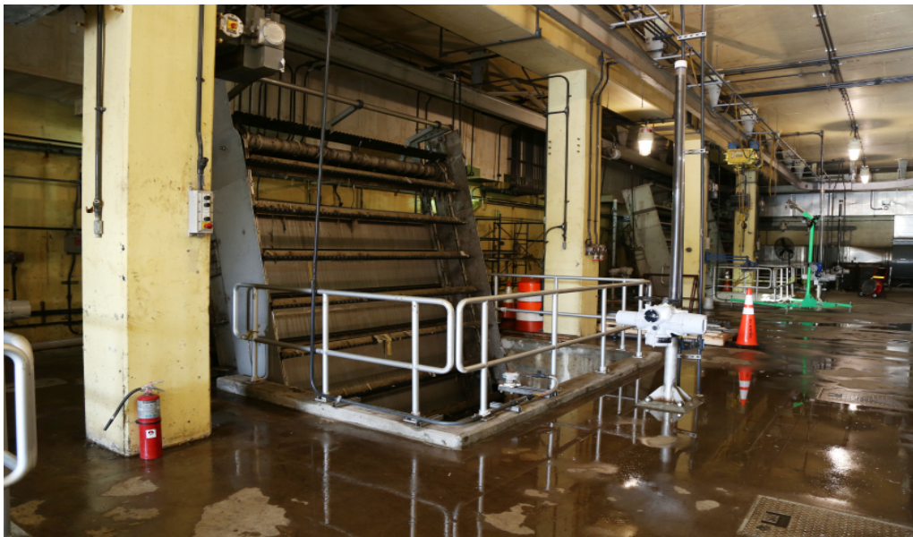
Potomac Pumping Station
