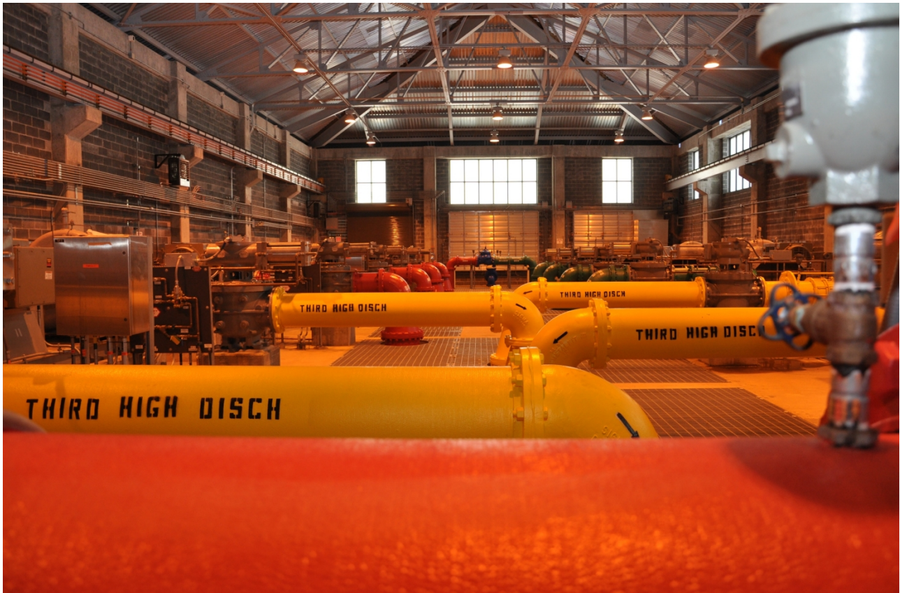
Anacostia Pump Station
