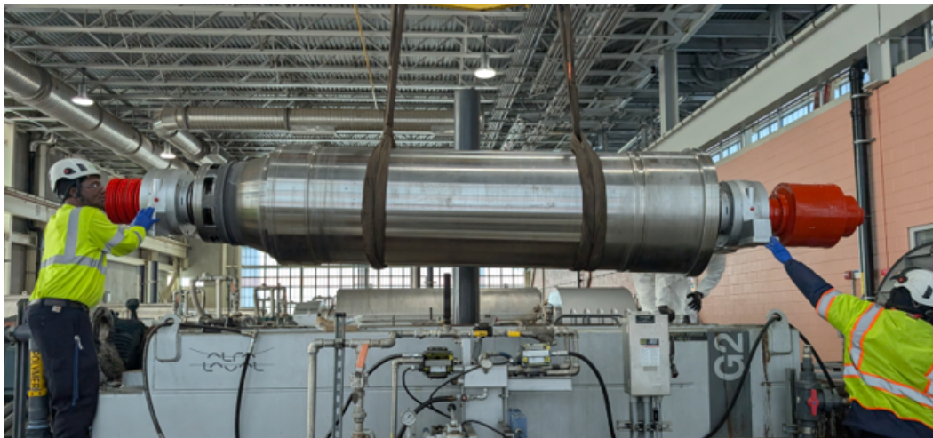
The picture shows DC Water staff aligning a large stainless-steel mechanical component part of wastewater treatment solids-processing equipment inside a maintenance facility. This highlights the heavy-duty equipment and precision mechanical work required to maintain DC Water's process engineering operations
