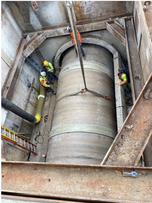
(Photo 1): Shows a typical launch and receiving pit where new pipe segments are pushed into the existing sewer pipe.
