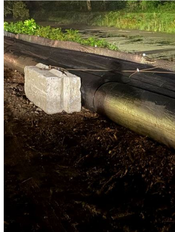
Bypass pipe secured with and blocks
