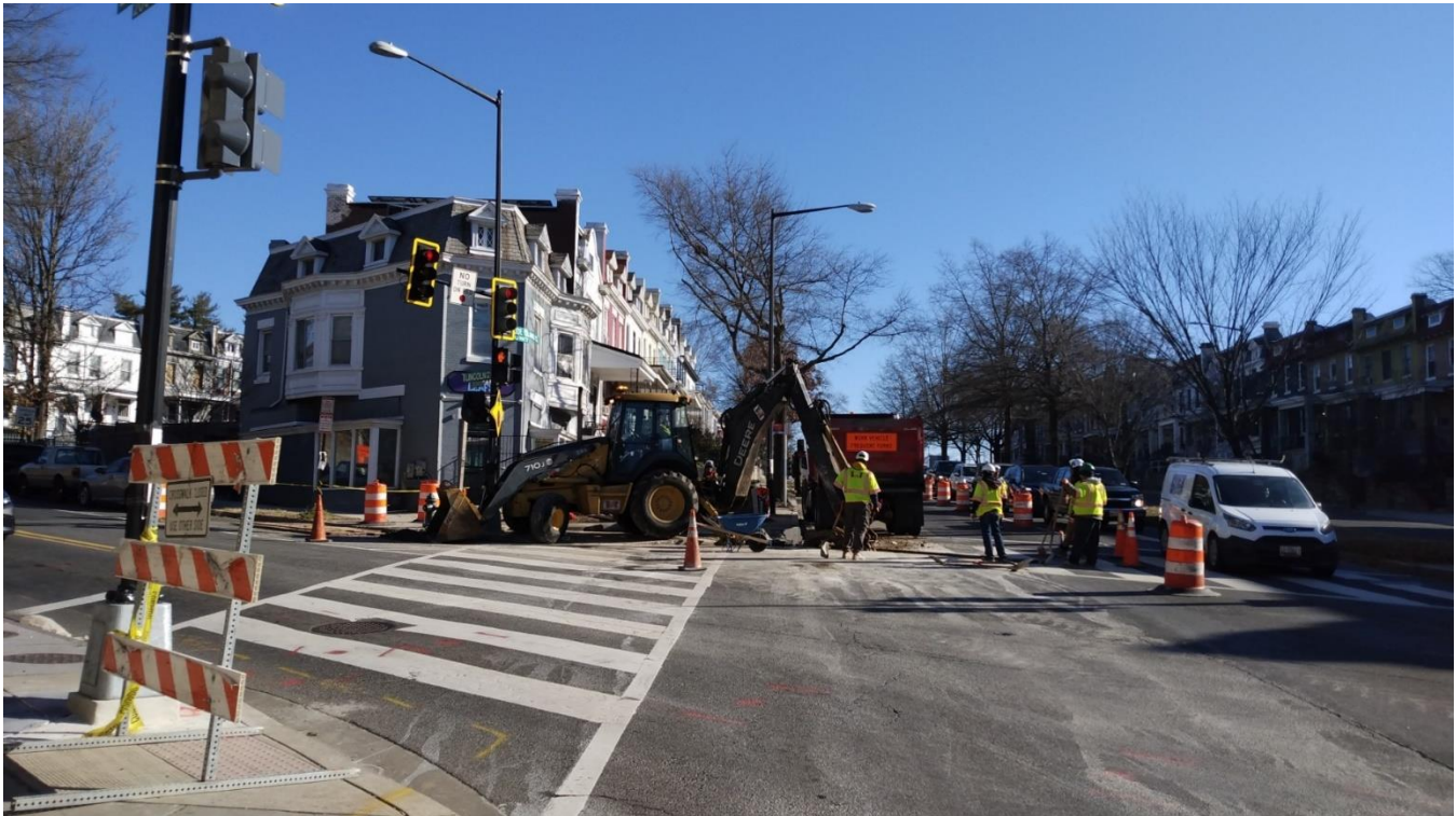
Traffic signal work in the westbound lanes of Rhode Island Avenue NE at the Lincoln Road NE intersection.
