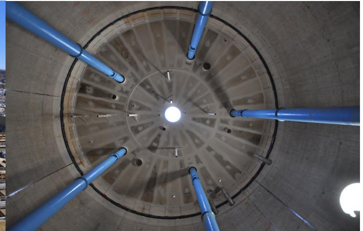
Inside View of Anaerobic Digester
