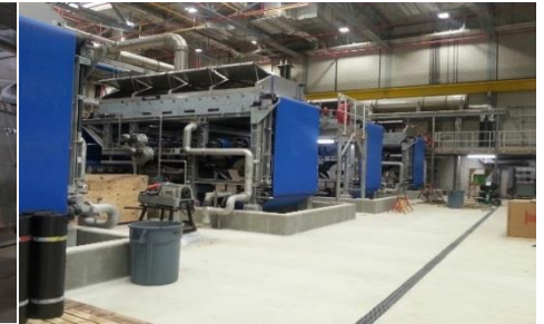
Belt Filter Presses
