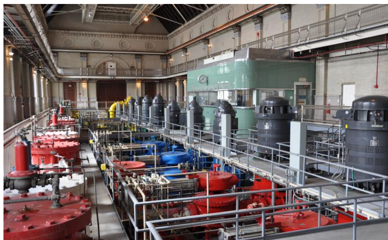
Bryant Street Pumping Station
