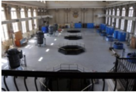
Main Pumping Station
