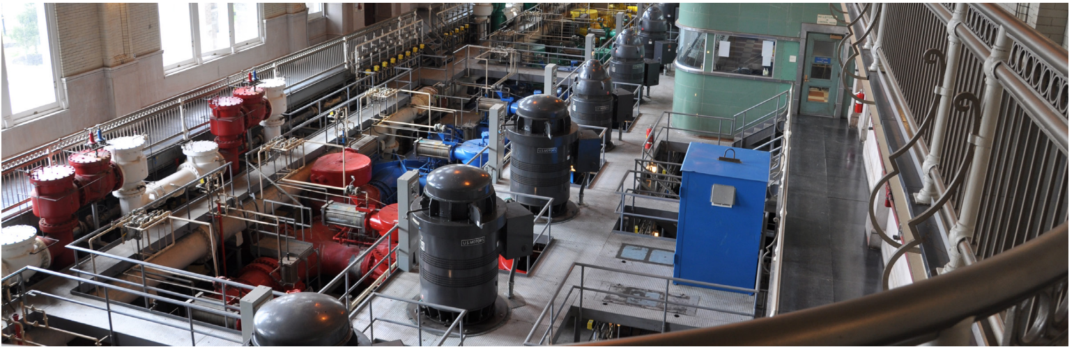
Bryant Street Water Pumping Station
