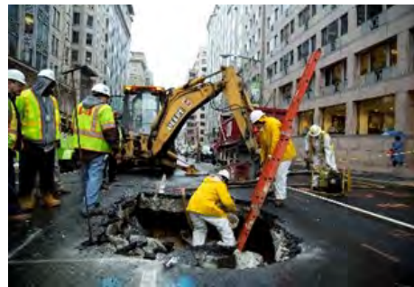
12th Street Water Main Break
