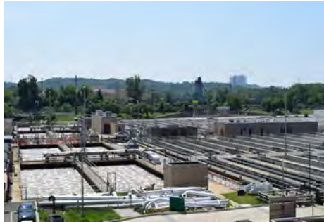
Blue Plains Advanced Wastewater Treatment Plant
