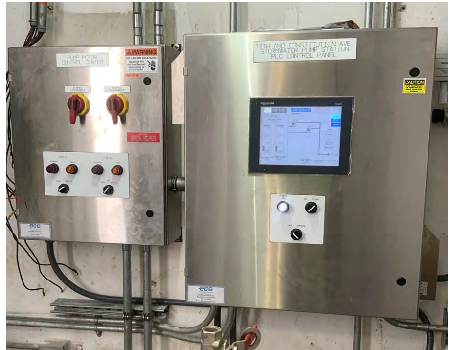
New SCADA Panels at Stormwater pump stations
