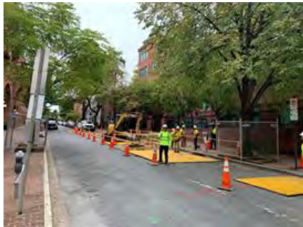
CSO-024 Manhole and Duct Bank
