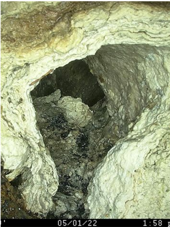
clogged sewer lateral (5/22)
