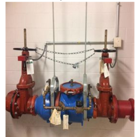
Backflow Prevention Assembly
