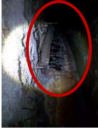
East West Outfall: Degradation of center wall
