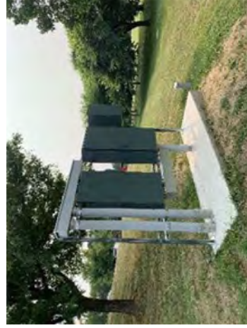
Electrical Panel at CSO 020
