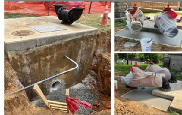
Emergency Booster Pumping – Ft. Reno PS
