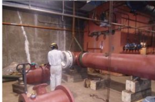
Reclaimed Final Effluent Pump Station Upgrades
