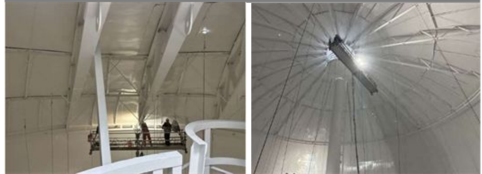
Anacostia Elevated Storage Tank No. 2
