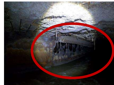
East West Outfall: Degradation of center wall
