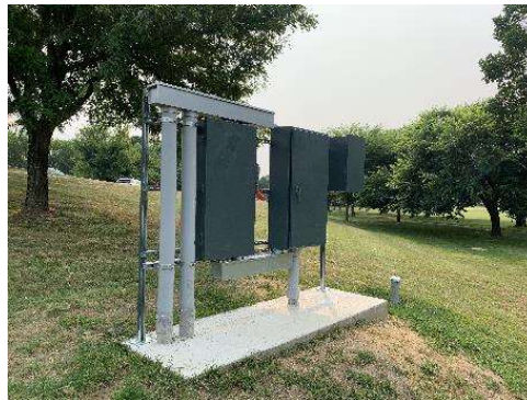
Electrical Panel at CSO 020
