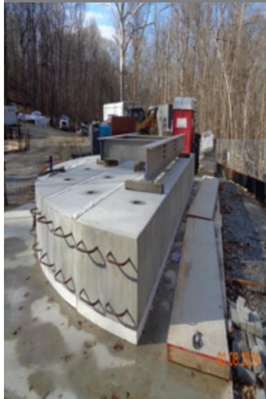
New MH31 Energy Dissipator
