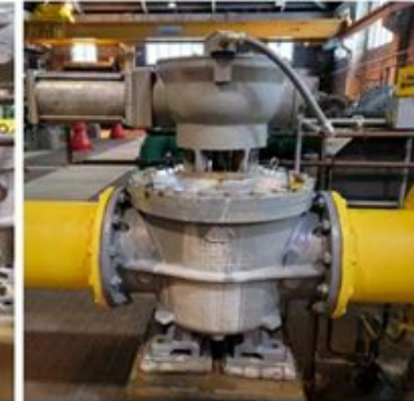
Figure C.14: Cone Valve at P12 – Packing Leak
