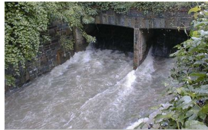
CSO 049 During Wet Weather Overflow
