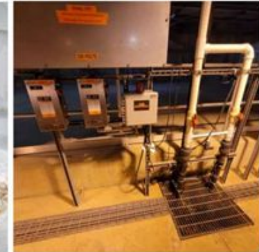
Figure C.26: Sump Pump SP-1 and SP-2
