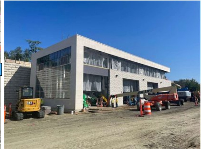
Ventilation Control Facility
