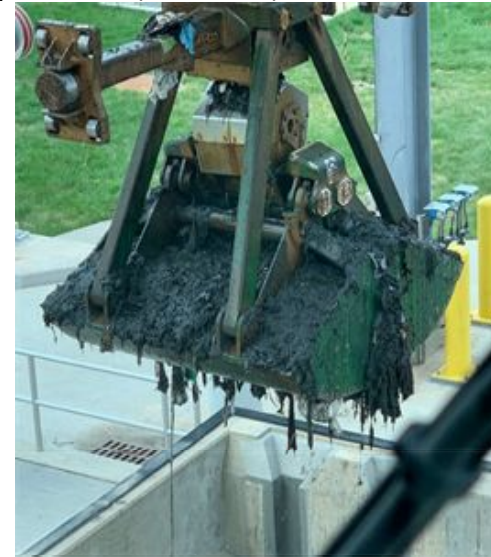
Trash, Debris and Solids Removal from Screening Shaft at Tunnel Dewatering Pumping Station
