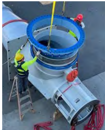
Filtrate Influent Pump Project
