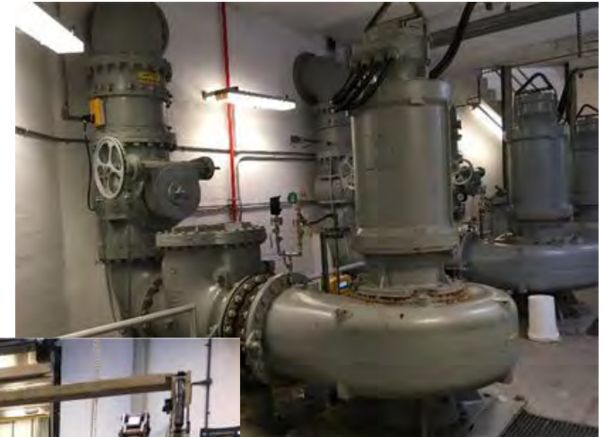
Rock Creek Pump Station
