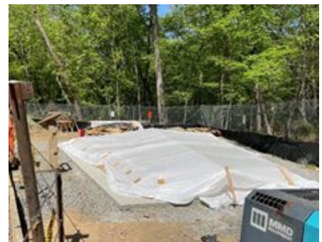
Concrete working pad to be used for upcoming formwork and concrete pour of CIP Roof Planks for MH31.5
