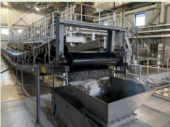
DC Water's fine screens capture solids
