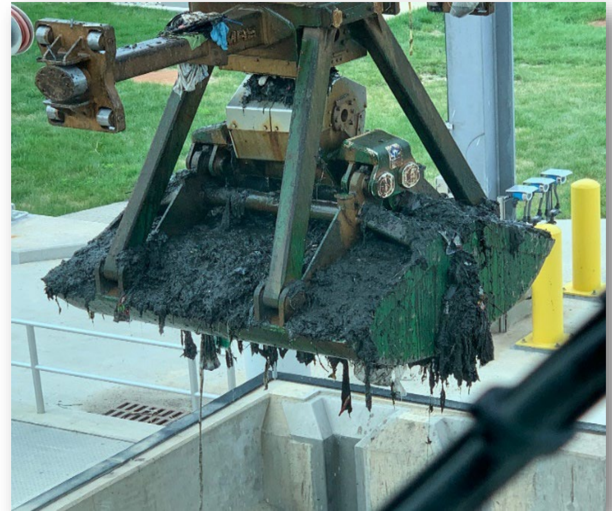
Trash, Debris and Solids Removed at Blue Plains from Anacostia Tunnel System
