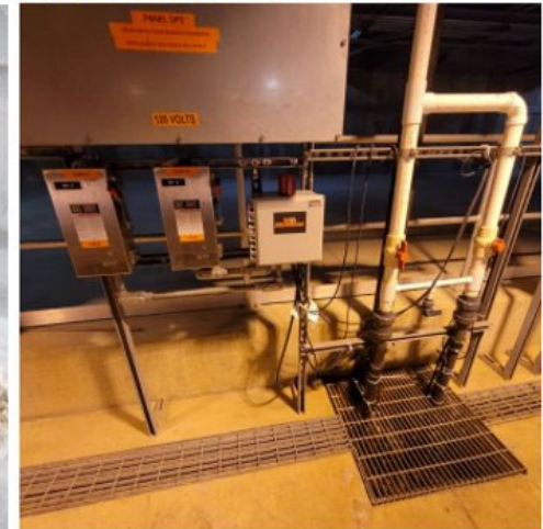
Figure C.26: Sump Pump SP-1 and SP-2
