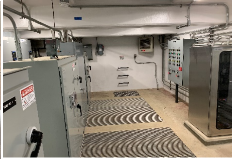
Stormwater Overflow Control Room
