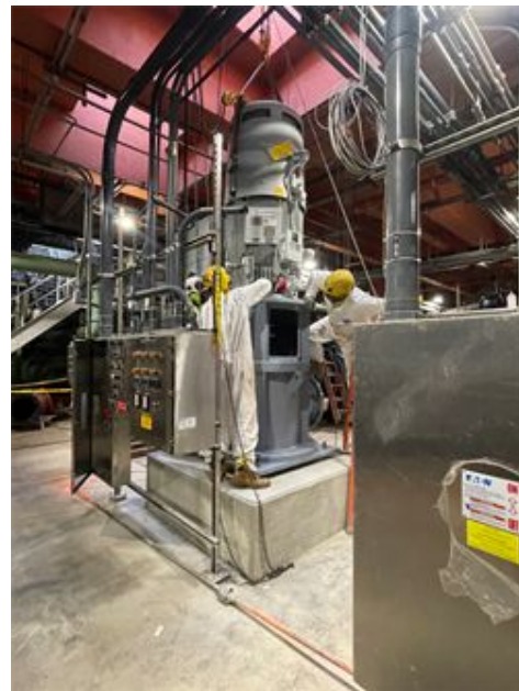
Contractor Ulliman Schutte (USC) mounting LPRFEP-2 motor from the FADF rooftop deck.
