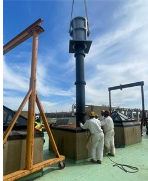
Contractor Ulliman Schutte (USC) with the assistance of United Crane Rentals delivering LPRFEP-2 via hydraulic crane to the FADF rooftop deck.
