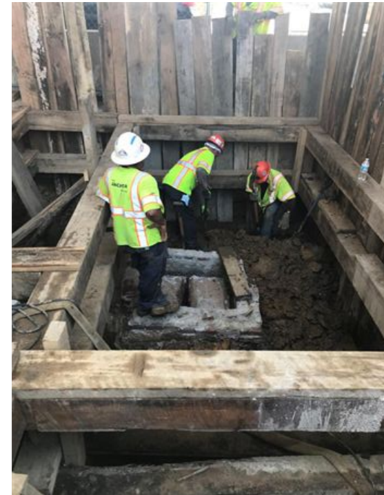
Excavation for Manhole 7 Connection to the Upper Potomac Interceptor at Wisconsin Avenue and K Street
