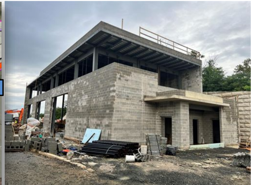
Ventilation Control Facility
